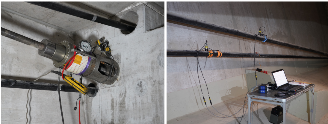
Figure 5.9: Experimental direct and indirect tension force identification: Lift-off test jack in place at span anchor (left) and vibration signal acquisition setup near the deviation block (right).
