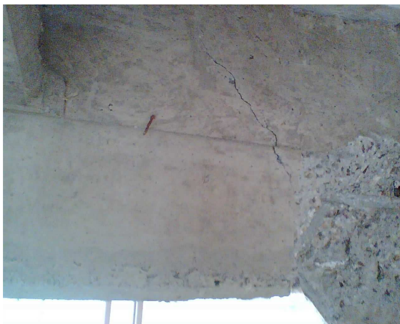
Fig.3. Cracked beam bracket
