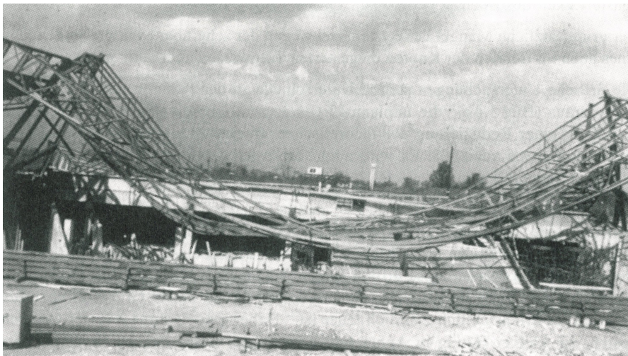
(c) Failure of truss girders, [61]
