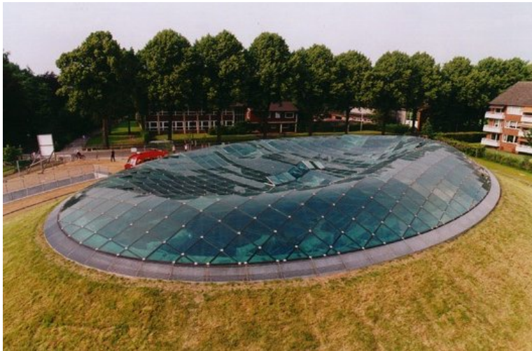
(a) Damage of the gymnasium in Halstenbeck, [10]
