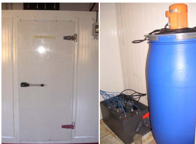
Fig. 5.3: Illustration of manure storage facility
