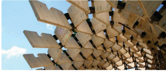
Fig. 4: structure with prepared integration of the gutters in the profile of the timber panels
